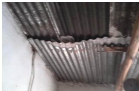
Fig. 5a: Homestead roofing attacked by termites
